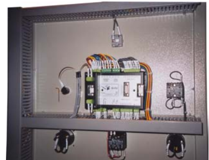
AMF panel, front door rear view
