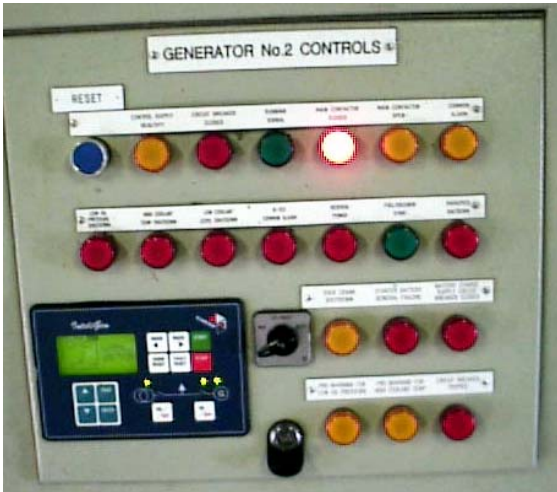
Modified control panel
